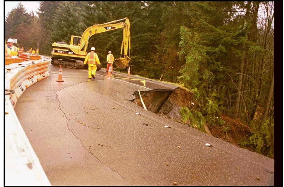
US 101 west of Olympia, M6.7 Nisqually Earthquake, 2001
