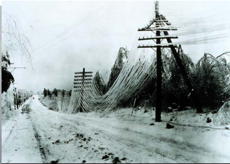
Power and telephone lines sagging after heavy ice storm
